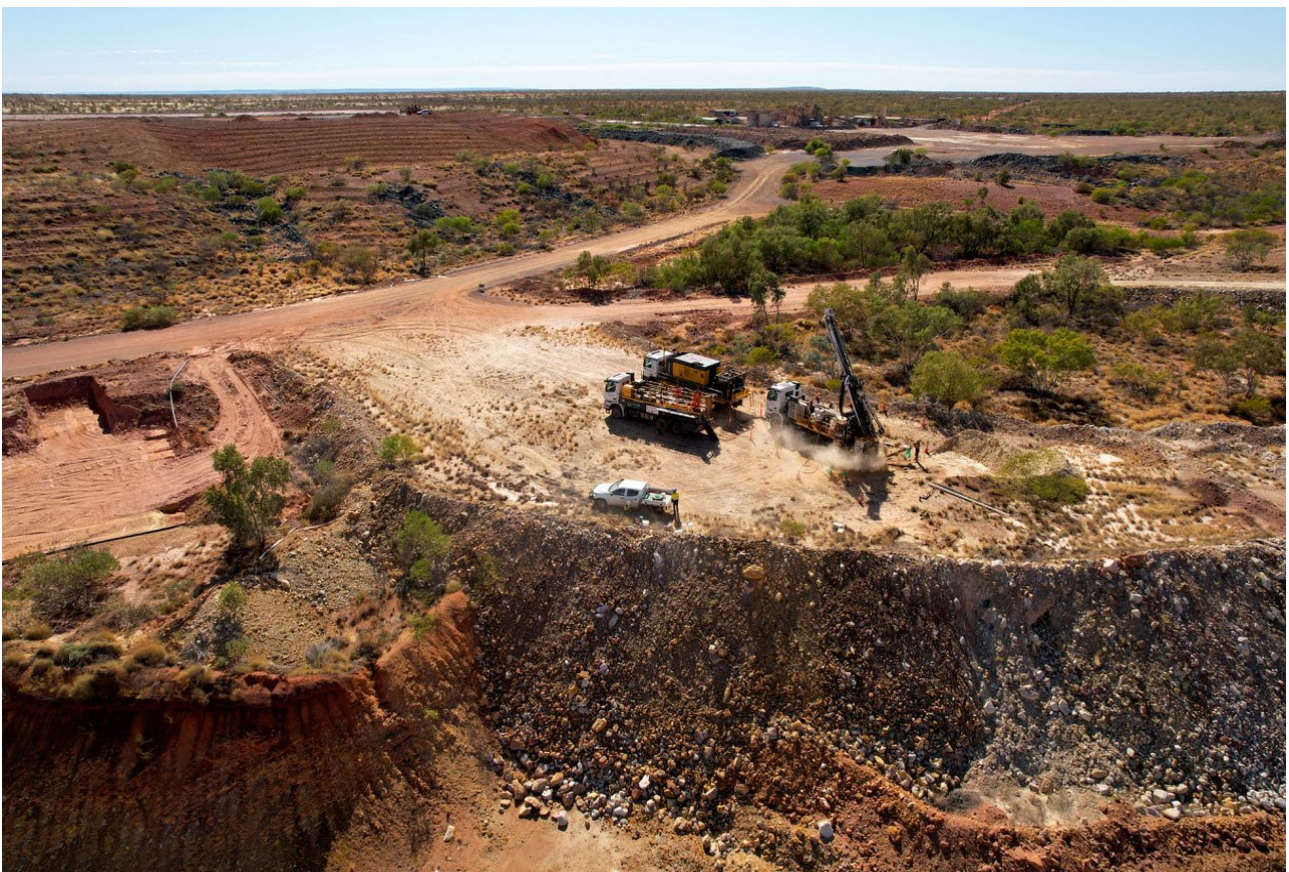
Figure 3: RC drilling for the extension and upgrade of the Speedy open pit Resource with ROM stockpiles, processing facility and camp in the background
