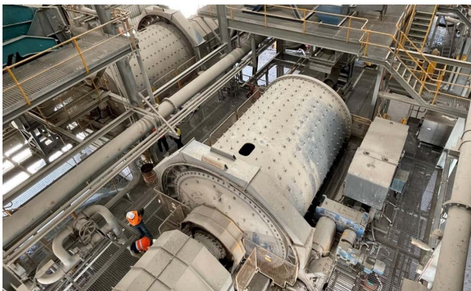
Figure 1: 1.85MW (foreground) and 1.45MW (background) Outokumpu ball mills with some of the associated infrastructure
