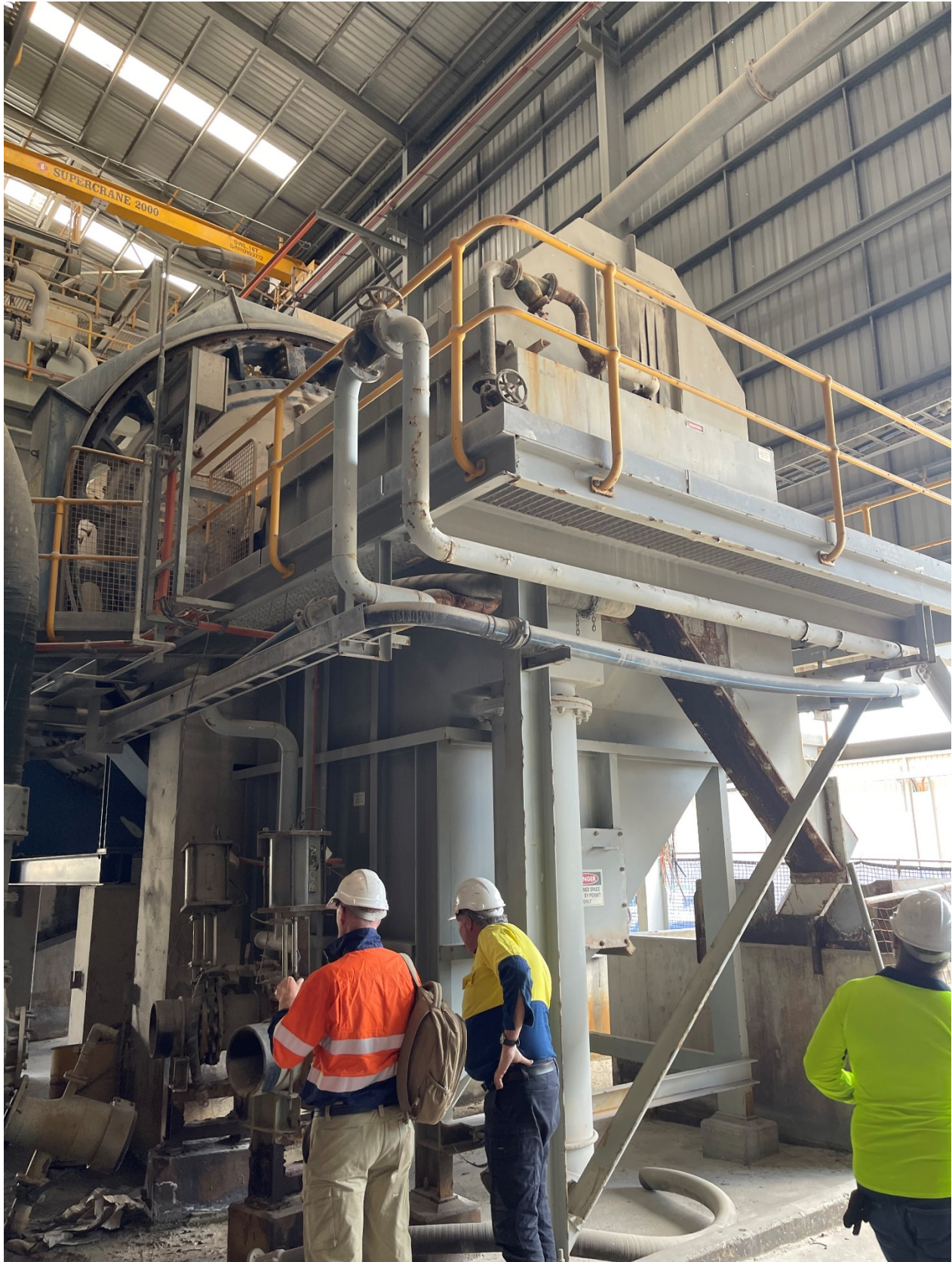
Figure 2: 1.45MW Outokumpu ball mill presently located in the South West of Western Australia
