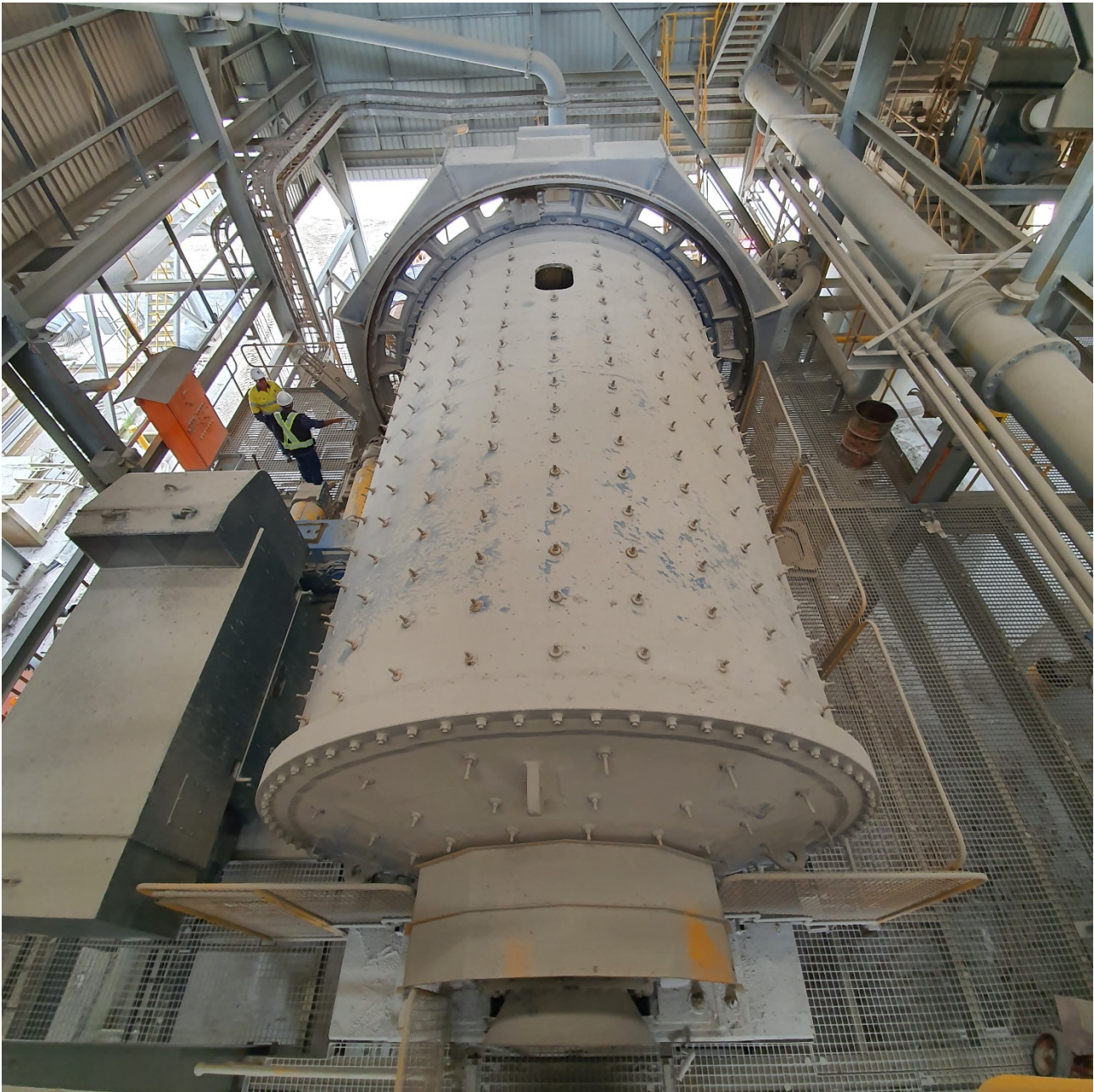
Figure 2: 1.85MW Outokumpu ball mill
