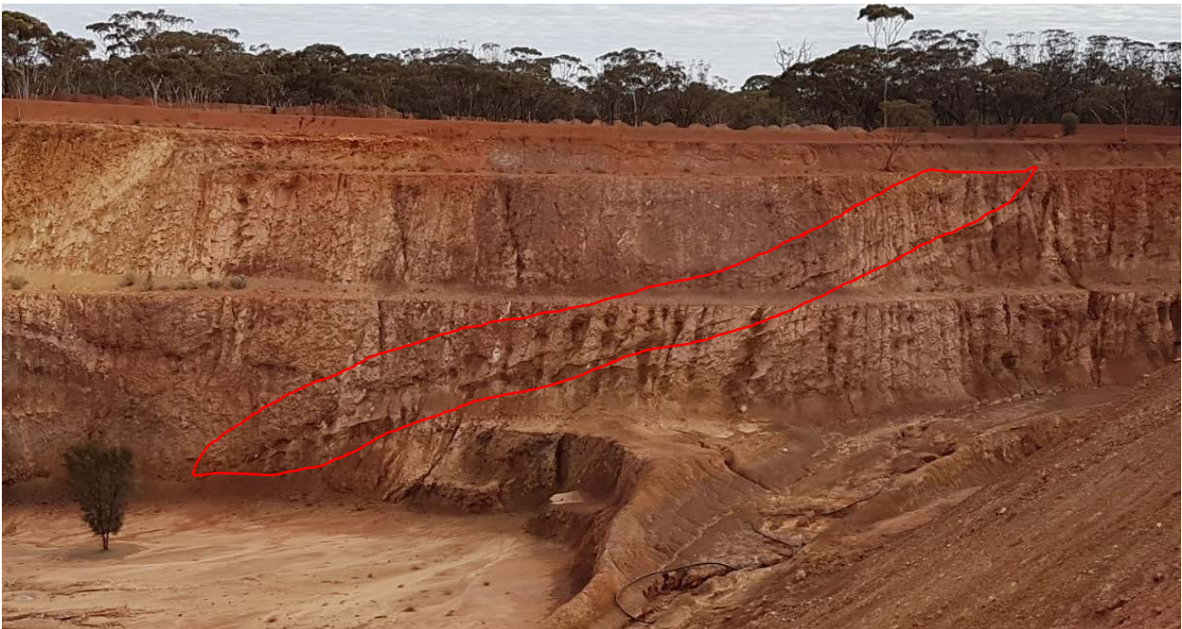
Figure 2: Photo looking at the north west wall of the Fingals Fortune open pit. Low angle veining is highlighted within the pit walls.
