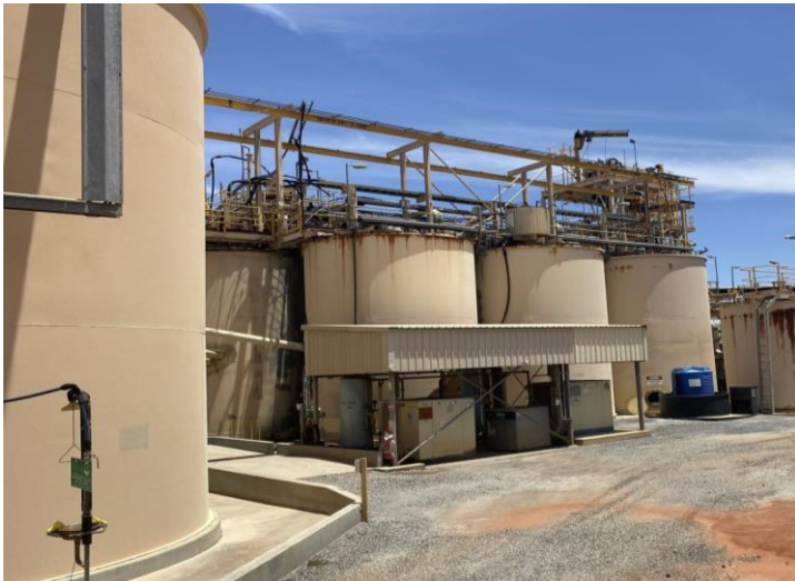
CIL tanks: 7x 150m 3 - steel ordered, agitators tested
